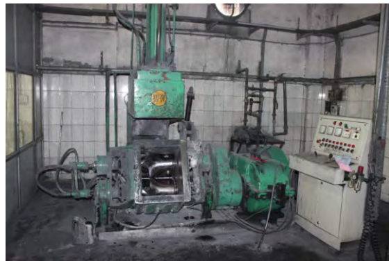
Fig. 1.5.2. Internal mixing shop floor
