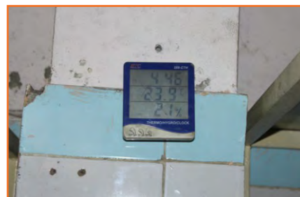
Fig. 4.1.3 Temperature & humidity control
