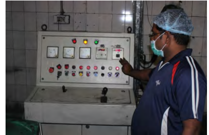
Fig. 3.1.3 Checking Control Panel settings
